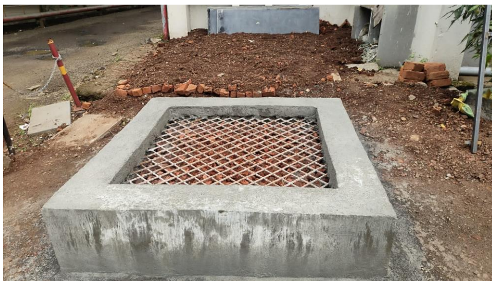
Photograph No.3 Showing Rainwater Recharge Pit in the College Campus
