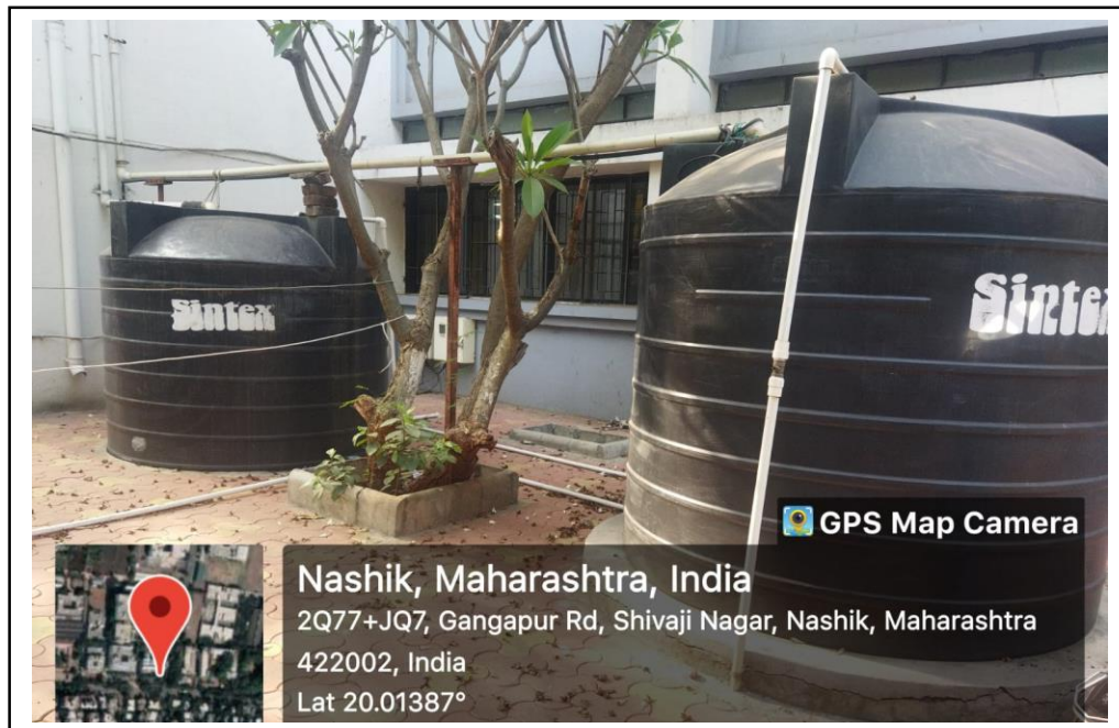
Water Storage Tanks
